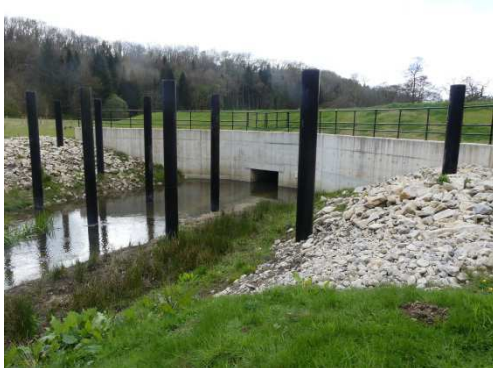
The concrete bund on the floodplain near Blansby Park, north of Pickering, designed as a water storage feature
